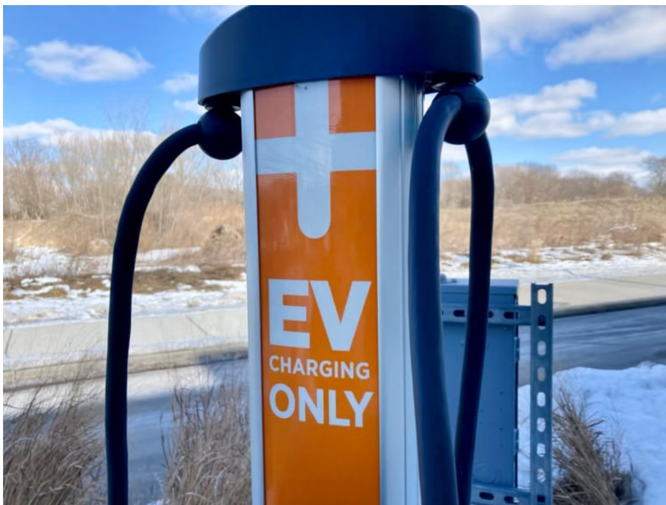
A ChargePoint electric car charging station sits in the parking lot of Garver Feed Mill in Madison, Wis., on Feb. 12, 2022. (Jim Malewitz / Wisconsin Watch)
